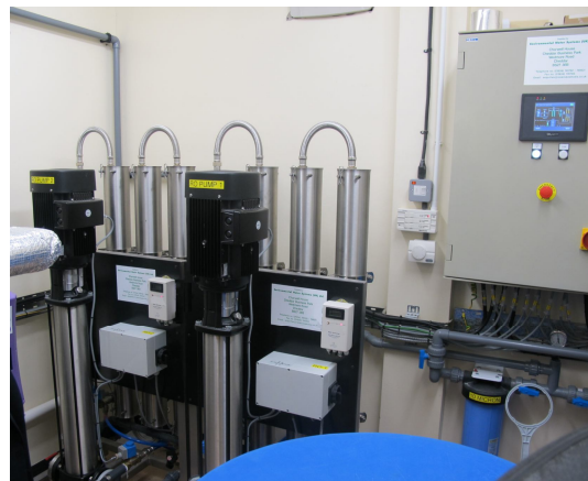
Thermal Sanitised RO Plant
