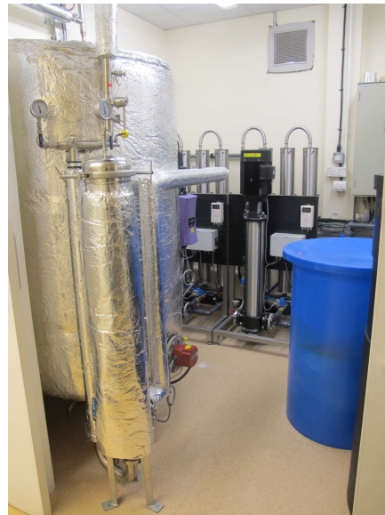
Compact RO Plant Room
