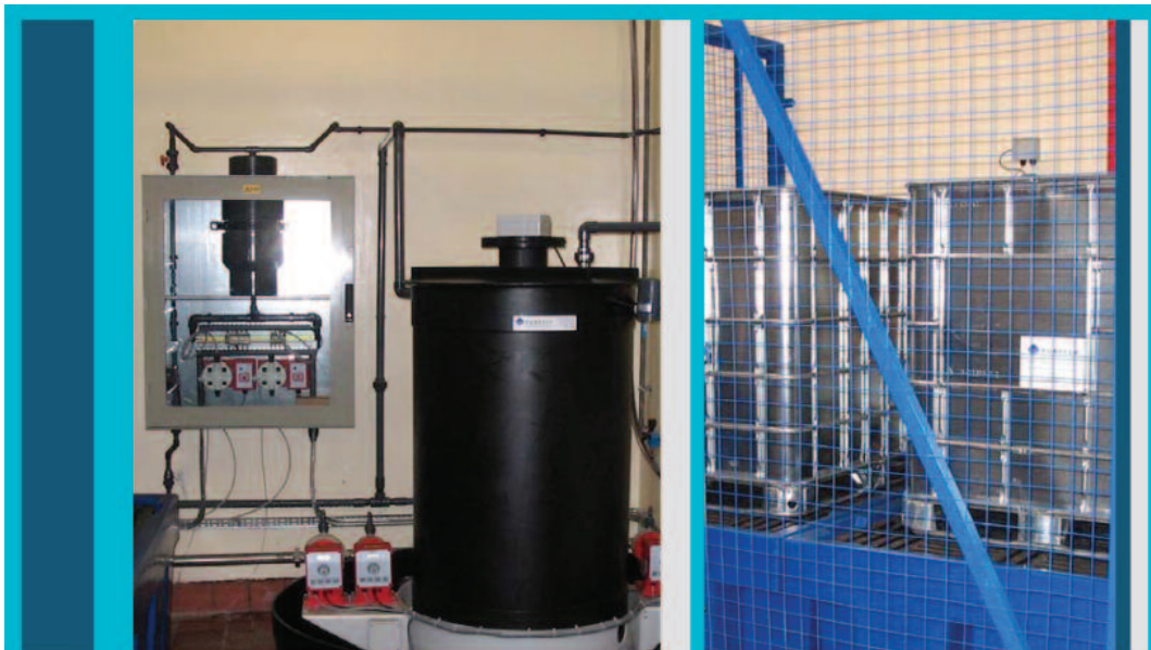
PureChlor Chlorine Dioxide Plant
