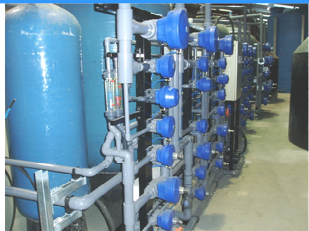
Part of the installation at Colour Anodising in Radcliffe
